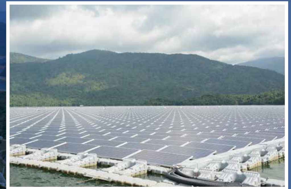
Floating Solar Power plant on Da Mi reservoir
